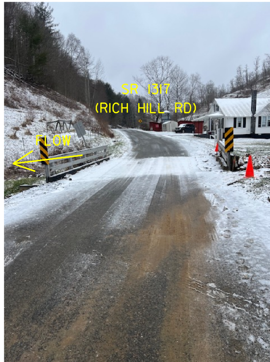
PHOTO #1: VIEW FACING NORTHWEST TOWARD END BENT NO. 1 FROM THE VICINITY OF END BENT NO. 2.
